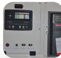
Control Panel & MCB
